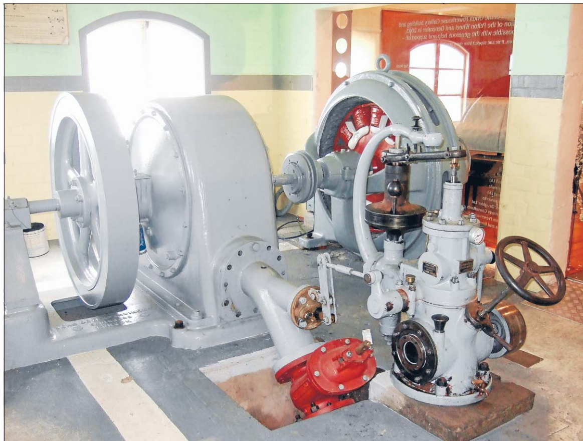
Restored: Akaroa's reconditioned 1908 pelton wheel power plant, repainted in its original colours and almost ready to generate electricity again.
