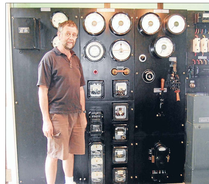
Labour of love: Electrical engineer John Dodgshun with the plant's control panel that he has rebuilt using historic switches and dials.
